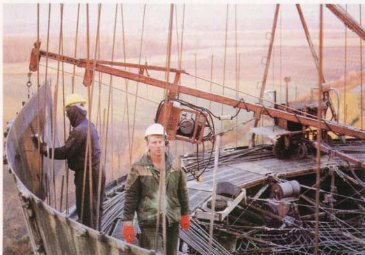
JIB CRANE is used to adjust form. Concrete and rebar were brought up by electric hoist.
